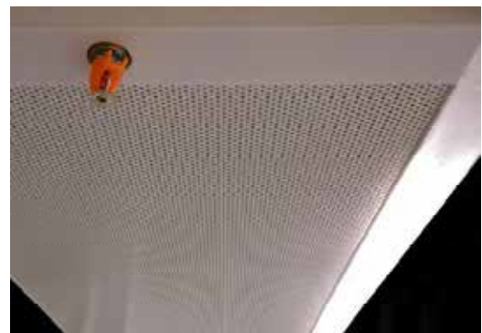
BOTTOM FACE OF PLENUM MODULE SHOWN WITH SPRINKLER AND LIGHTS
