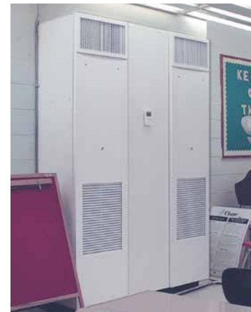
Custom side-by-side exposed installation
