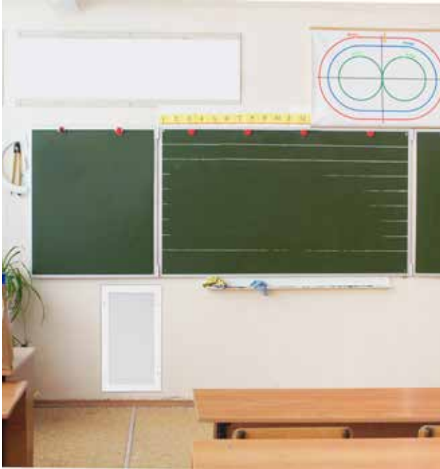
Example of an internal wall mounted diffuser.
