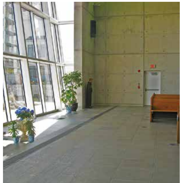
Example of a floor mounted diffuser.
